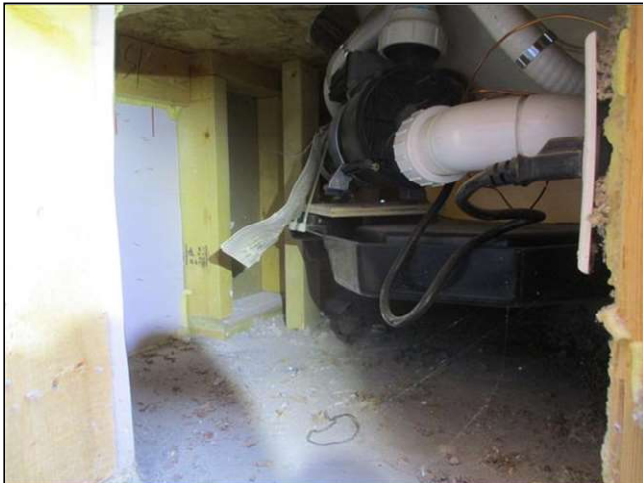
Tub pump motor access on West side
