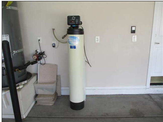
Water softener is not inspected
