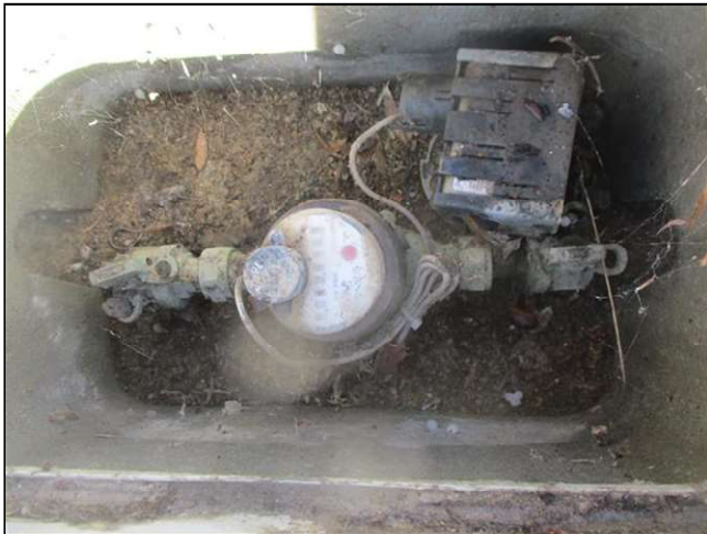
Water meter / main shut-off
